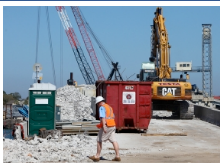
Workers continue to remove concrete from the temporary bridge on Friday. The rubble will be used to stabilize the old Iberia Street landfill. By DARON DEAN, daron.dean@staugustine.com.
